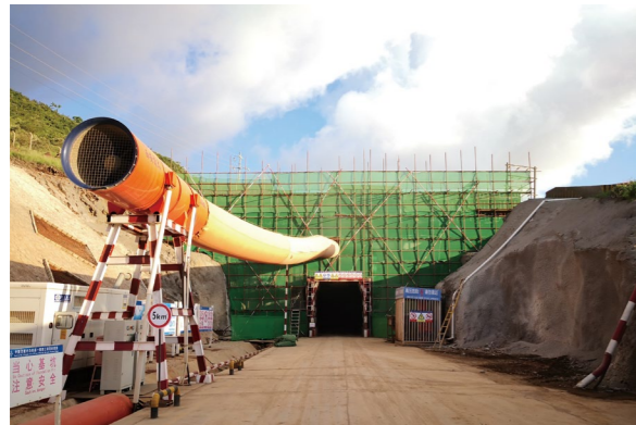
隧道通风降尘设备 Tunnel ventilation and dust control equipment
